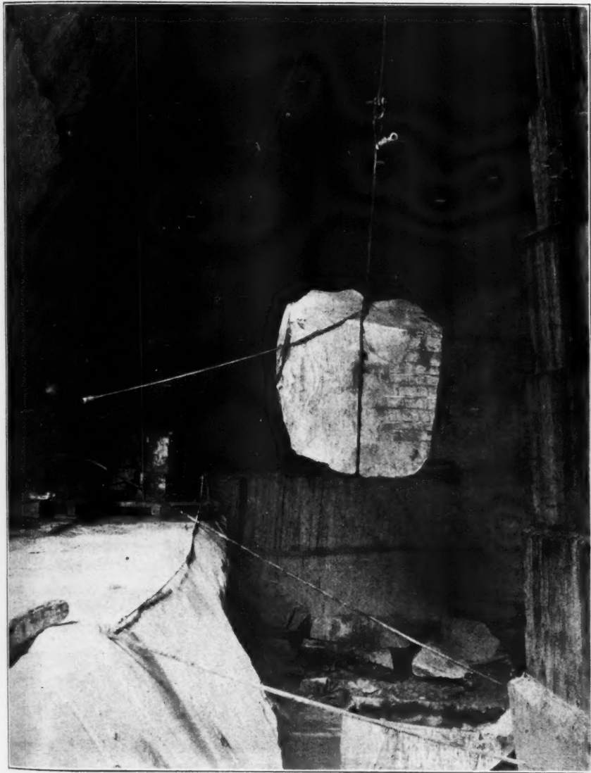
Block of Marble Being Lifted From the Bottom of Tunnel By Derrick
